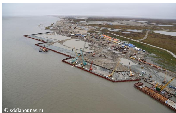
Figure 4.50 The 975-metres long quay wall of the Sabetta seaport is constructed to receive cargo to build Yamal LNG and to ship its production in the future.
