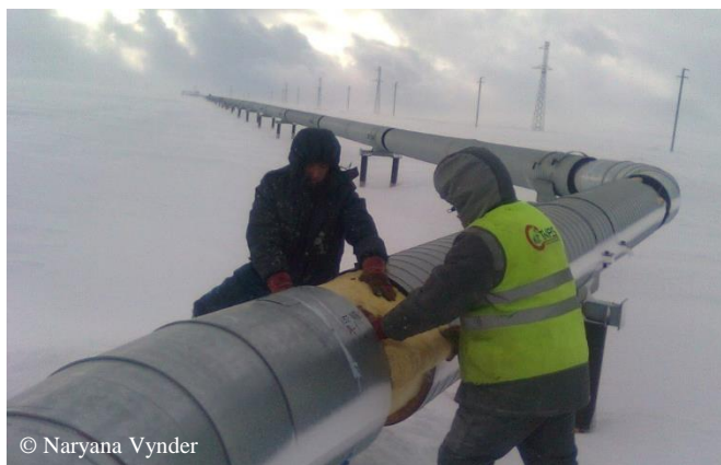
© Naryana Vynder Figure 4.58 Oil produced at big oil fields named after Roman Trebs and Anatoly Titov will be shipped via the Varandey terminal. Photo: construction of a 43-kilometres pipeline connecting two oil fields.
