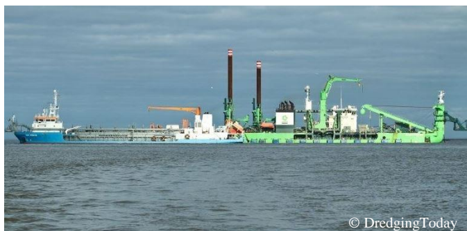
Figure 4.49 A 50-kilometres long sea channel is being built in the Ob Bay to approach the Sabetta seaport. The volume of dredging works will total about 70 million cubic metres. Photo: dredging operation in the Ob Bay in August 2014.
