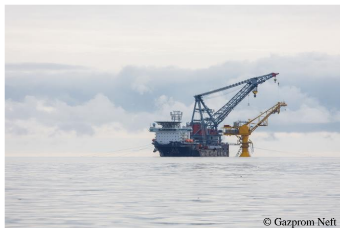
Figure 4.48 In 2015, Gazprom Neft completed pre-construction works of the Arctic terminal offshore in the Ob Bay. The terminal is designed for all-year-round operations and has a capacity of 8.5 million tonnes per year. Photo: Oleg Strashnov installing the oil offloading tower at the Arctic terminal in the Ob Bay.
